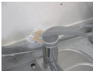
Fig. 6. Limit switch sensor on a faucet.
